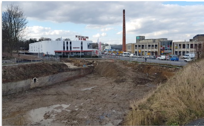
Fig 12. View from Hoge Fronten towards the Cabergerweg (14-03-2018). In the foreground the preparatory work for the underpass of Cabergerweg that will connect the fortifications of Hoge and Lage Fronten. (Source: KLEON3 at Wikimedia Commons).
