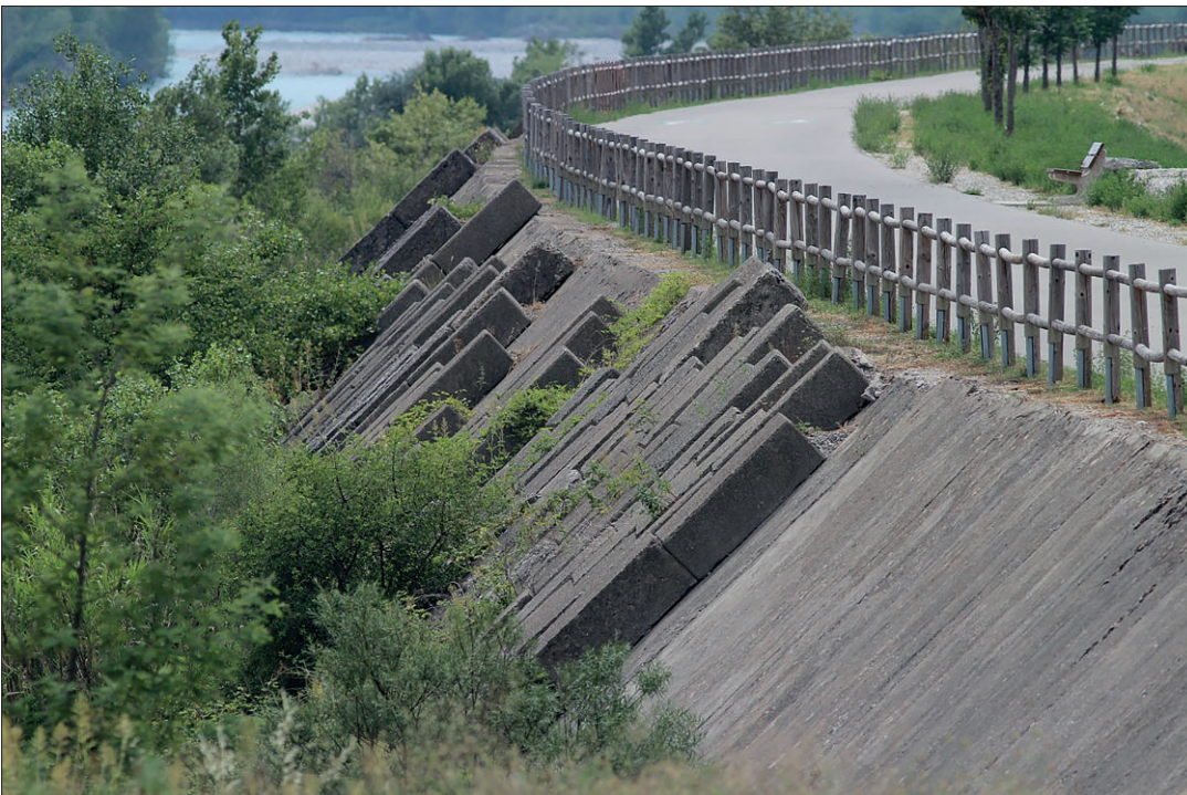
Figure 2 – View of the study site – Details of the dike with the blocs and cycle path (photo M. Belaud).
