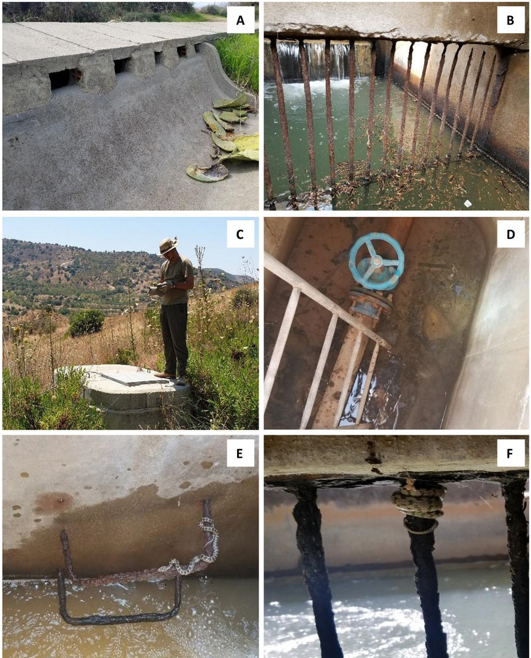
Figure 2. An overview of the outside and inside area (A and B) of the main sampling site, at the Kissonerga area. The concrete construct has openings to allow water overflow, and rusted metal bars inside the channel. Other artificial irrigation construct (e.g. the Marathounta 2 site) have narrower and deeper openings that are filling seasonally with water (C and D). Reptile species commonly found entrapped in the irrigation channel are the Hemorrhhis nummifer (E) and the Telioscopus fallax (F). Photos by Antreas Kourides.
